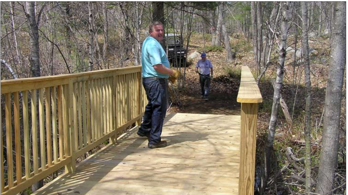
Bud Danis and Bill Case work on the new bridge at the Steele Trail.
